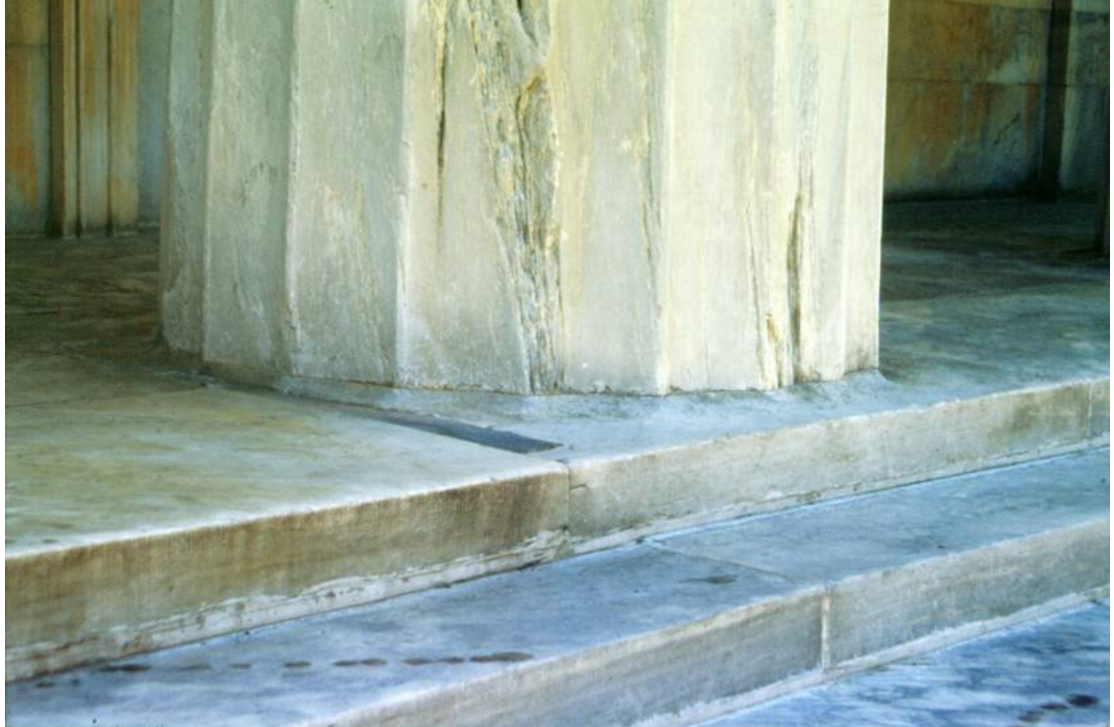
Fig. 22 Philadelphia, PA. Second Bank of the United States. Drum of marble column set on the floor as in antiquity.
