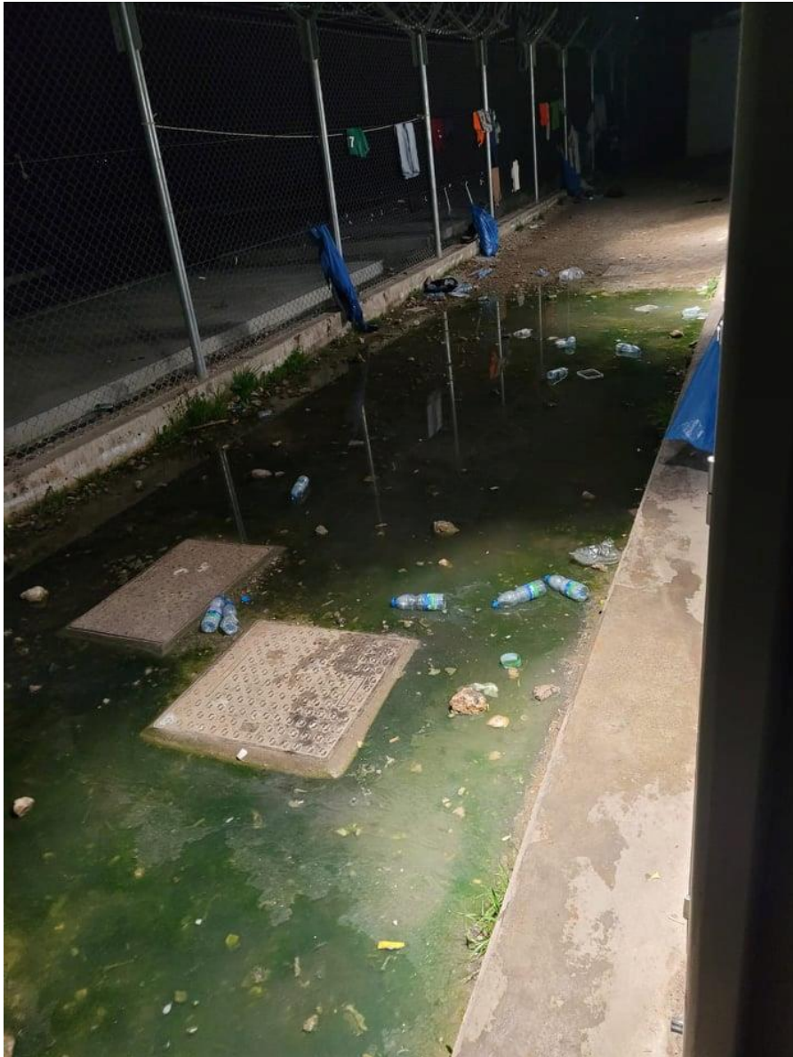
Picture from the sewers flooding in Pournara
